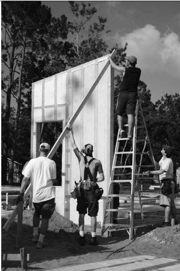
Students begin to set up the modular panels of the preHAB house in Gautier, Mississippi.
