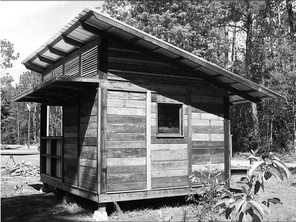
The siding, as seen on the west side of a shed built in June 2007 for Billy Ray Raines, is "barge-board" salvaged from New Orleans houses. The 2- by 6-inch posts and beams are from a deconstructed Ocean Springs, Mississippi, home. Photo credit: Brad Guy.
