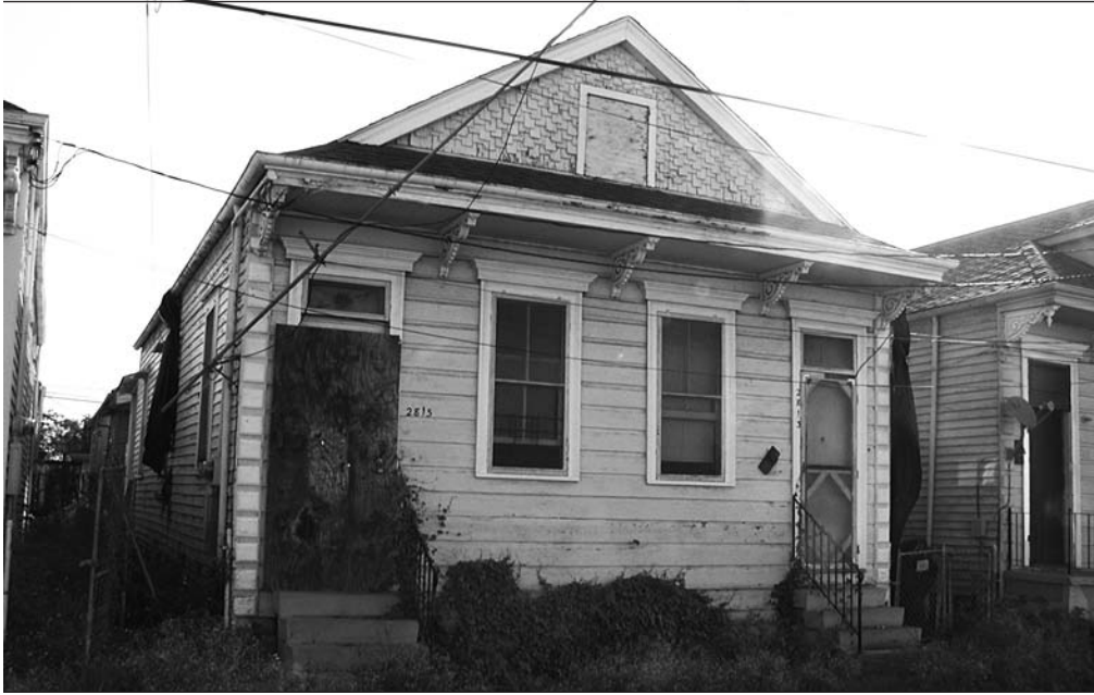
A typical duplex unit in the Tremé/Lafitte neighborhoods in Orleans Parish, with the water line from Hurricane Katrina flooding visible on the fourth row of siding. Photo credit: James Goedert.
