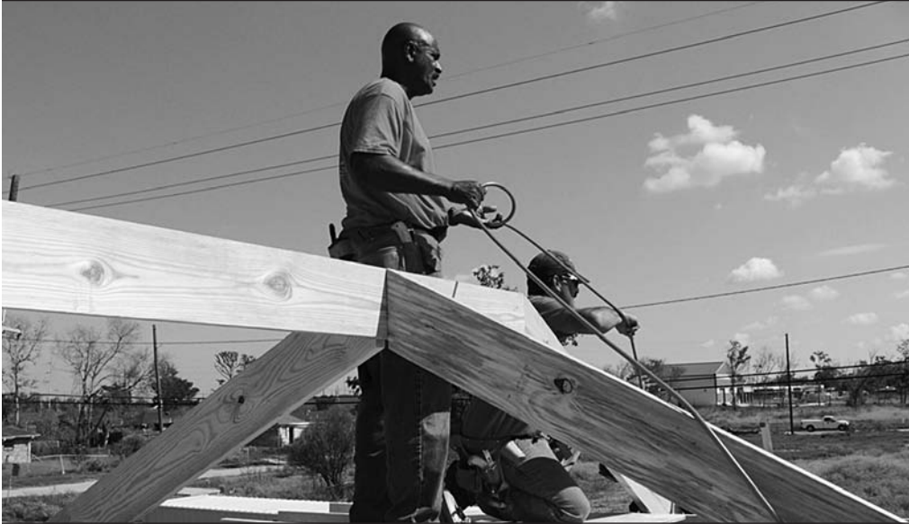
Pastor Melvin Jones, founder of Bethel Colony South, oversees the roof framing of the House at 2310 Delery Street, Lower 9 neighborhood, New Orleans. Photo credit: Marsha Cuddeback.
