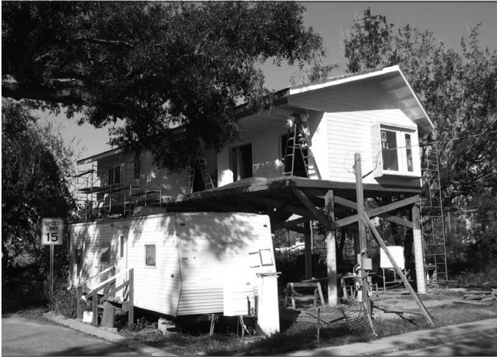
Patricia Broussard's new East Biloxi house rises behind the Federal Emergency Management Agency's (FEMA's) trailer in which she has lived since Hurricane Katrina damaged her home. Photo credit: Vincent Baudoin.
