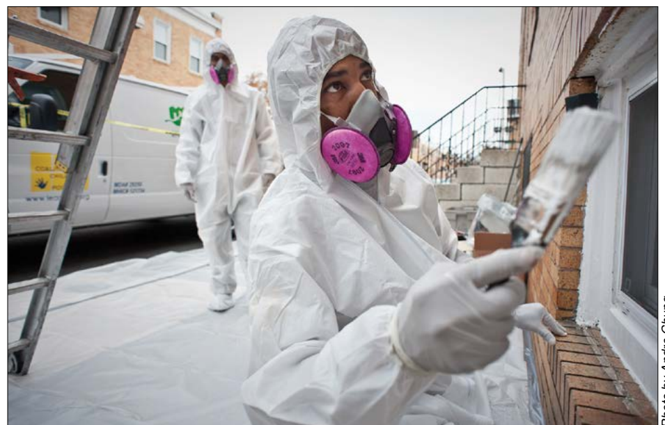
A GHHI hazard reduction worker paints a new lead-free window frame. Although much progress has been made toward reducing instances of lead poisoning, an estimated 22 percent of homes have one or more lead-based paint hazards.
