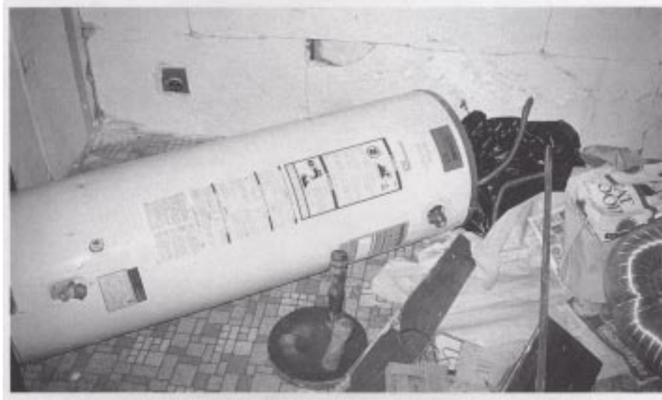
Figure 30. An example of frequent damage to water heaters.
