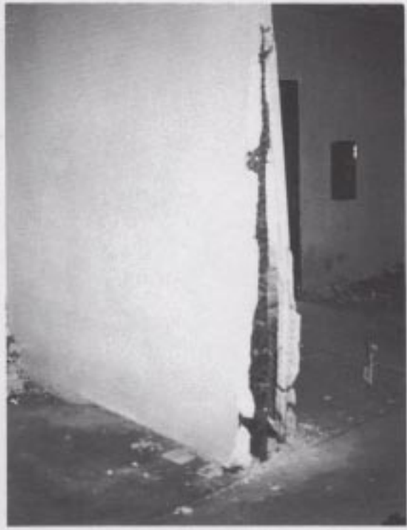
Figure 53. A damaged stucco and wood-frame narrow shear wall located on the first story of an old garden-apartment complex.
