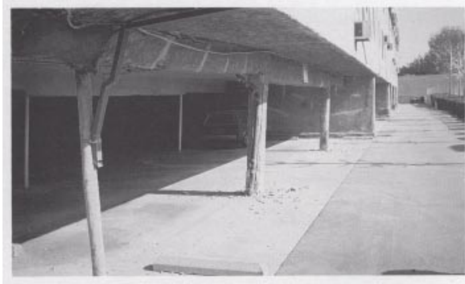
Figure 62. An older soft-story foundation supported by stucco shear walls on one end and steel pipe columns on the other end (near side) creating an imbalance in lateral stiffness.
