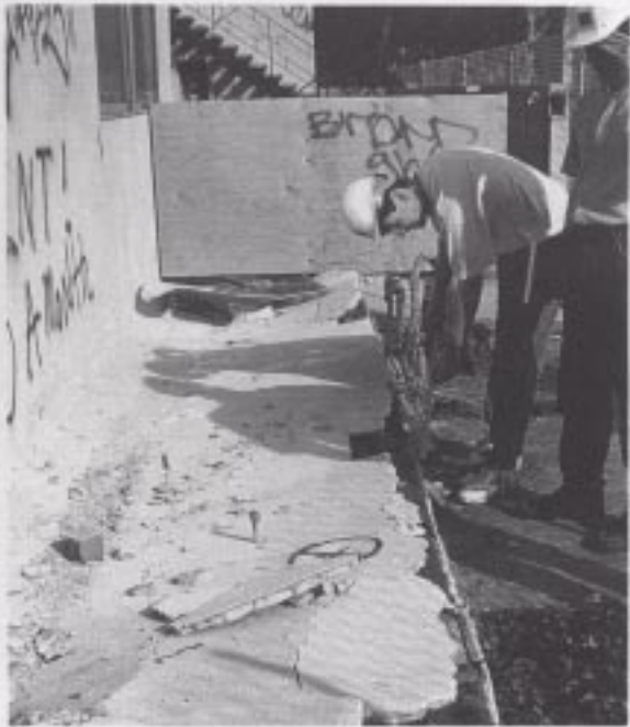
Figure 50. Collapse of a cripple-wall foundation connected to a collapsed soft-story garage on Mammoth Avenue.
