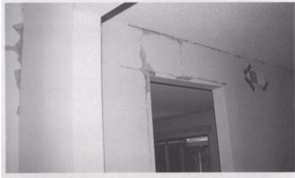
Figure 32. An example of severe (“HIGH”) interior finish damage (gypsum board) at partition wall intersections and openings in the walls.
