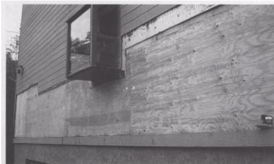
Figure 57. Newer MFLR construction showing the use of plywood sheathing on wood framing.
