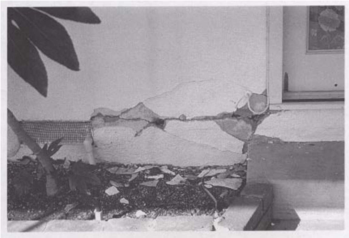
Figure 15. Stucco damage along the top of a crawlspace foundation on a SFD home.
