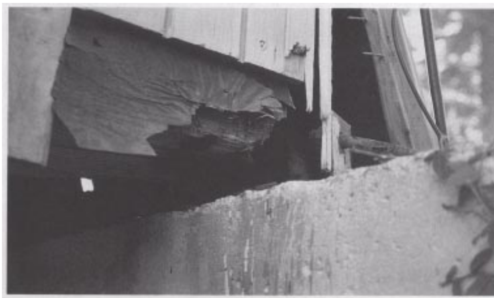
Figure 21. Example of a critical failure at the connection of the floor joists to the foundation wall on the same home as in Figure 20. (Foundation/wall connection rating: HIGH)
