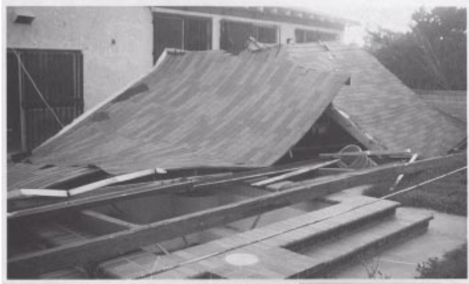
Figure 33. An infrequent collapse of a porch attached to a home.
