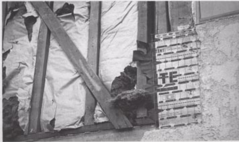
Figure 51. A damaged stucco and wood-frame wall under repair showing 3x framing and a 1x let-in brace disconnected from the sill plate.
