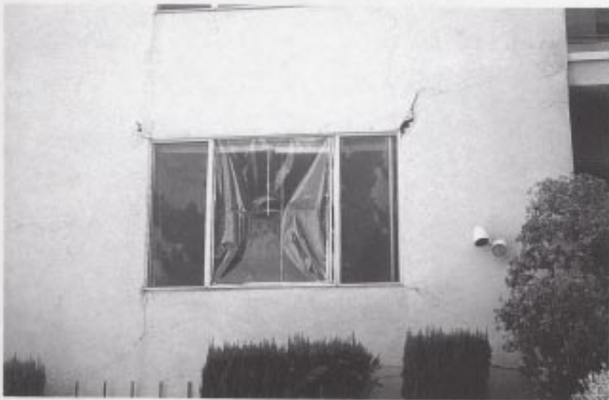
Figure 8. Photograph of a MFLR building with "MODERATE" damage to the First Story-Exterior Wall Finish (stucco) of a MFLR building.
