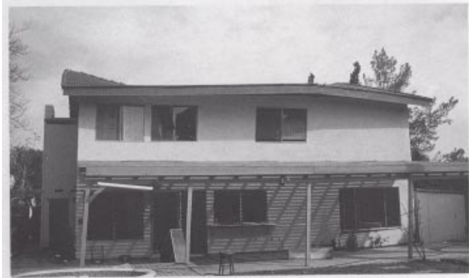
Figure 25. An example of severe roof damage on an overloaded gable-roof with heavy tile roofing. (Roof damage rating: HIGH)
