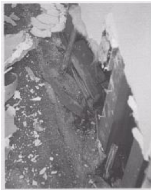
Figure 60. A view inside the building shown in Figure 59 that reveals a missing hold-down bracket, a sheared sill bolt, and a splintered sill plate.
