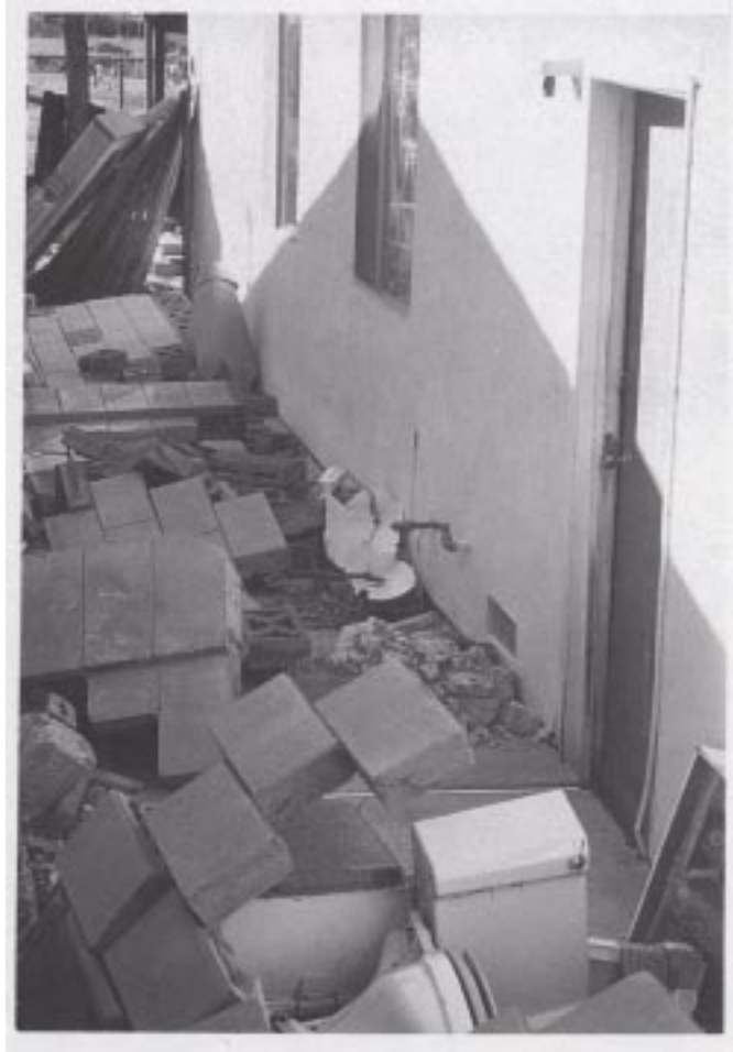
Figure 17. An example of one home in Simi Valley which experienced settlement because of soil liquefaction. (Foundation damage rating: HIGH)
