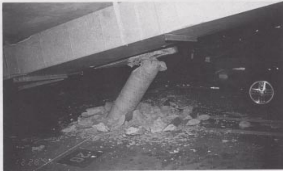
Figure 48. A view inside the collapsed garage showing a small, telescoped concrete column crushed by the weight of a thick concrete slab and added inertial load from potentially high vertical ground acceleration.
