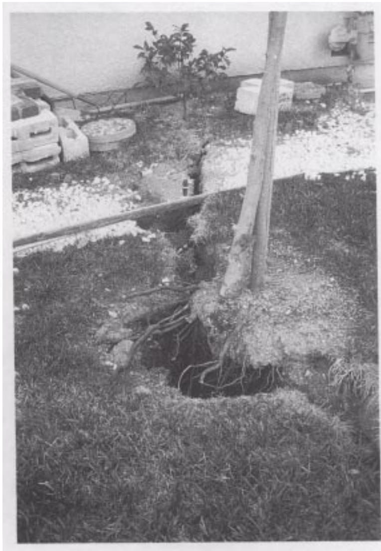
Figure 18. An example of a ground fissure intersecting the foundation of a home located in the Tujunga Canyon area.
