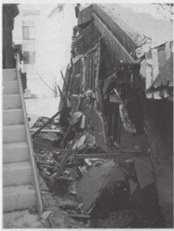
Figure 49. Separation and collapse of a soft-story garage area (right side) once connected to the unmoved portion supported by a slab-on-grade foundation (left side).
