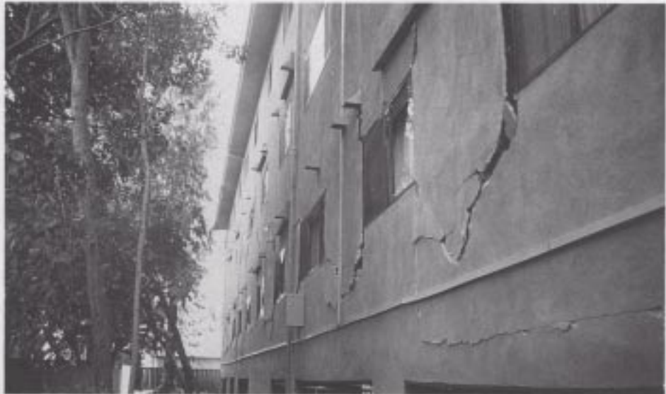
Figure 55. Severe shear cracks in stucco finishes between window openings and along the top of the garage foundation.
