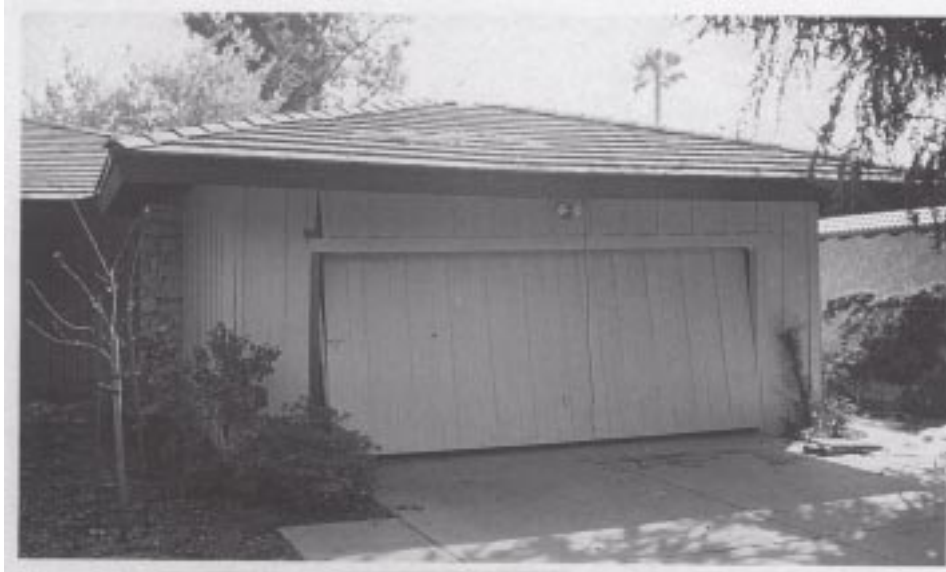
Figure 24. An example of wall racking resulting in damage to a garage door opening. (Wall damage rating: HIGH)
