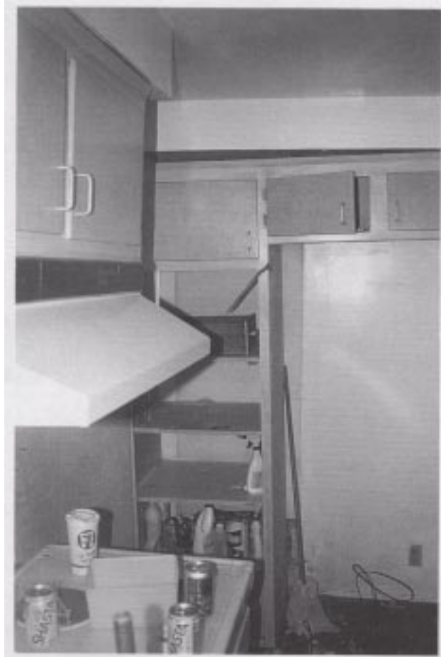
Figure 29. An example of damage to shelves and cabinets in the kitchen of one home.
