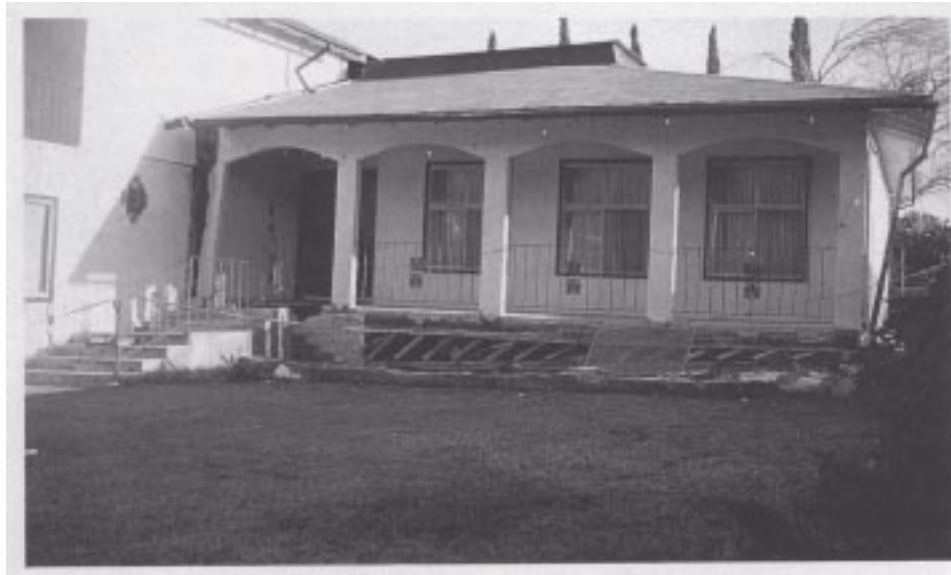
Figure 22. An example of a foundation collapse of the section of a home supported on a cripple wall caused by the 1994 Northridge Earthquake.
