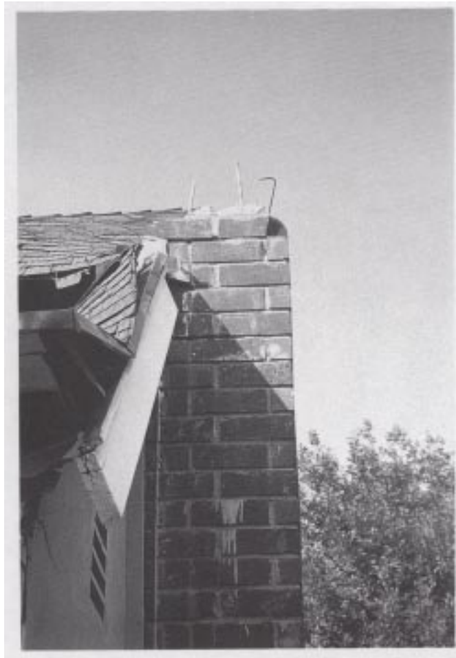
Figure 27. An example of damage to masonry chimneys and the surrounding roof framing.
