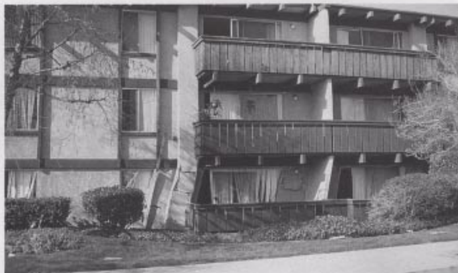
Figure 41. Another section of the Northridge Meadows MFLR building where the soft story is severely racked, but not collapsed.
