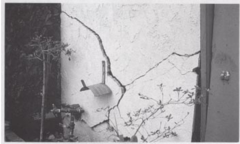
Figure 31. An example of severe stucco damage.
