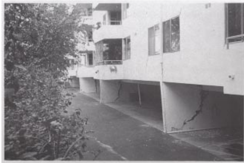
Figure 45. Failure and diagonal cracking of a wood-frame and stucco shear wall used in this soft-story MFLR construction.
