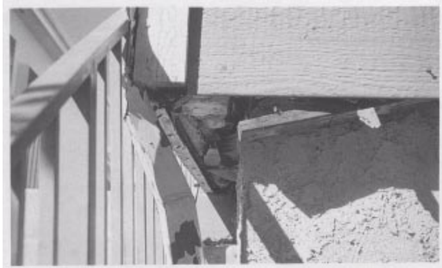
Figure 59. Fractured sill plate and sliding of a new MFLR building on top of an undamaged, reinforced concrete garage foundation.
