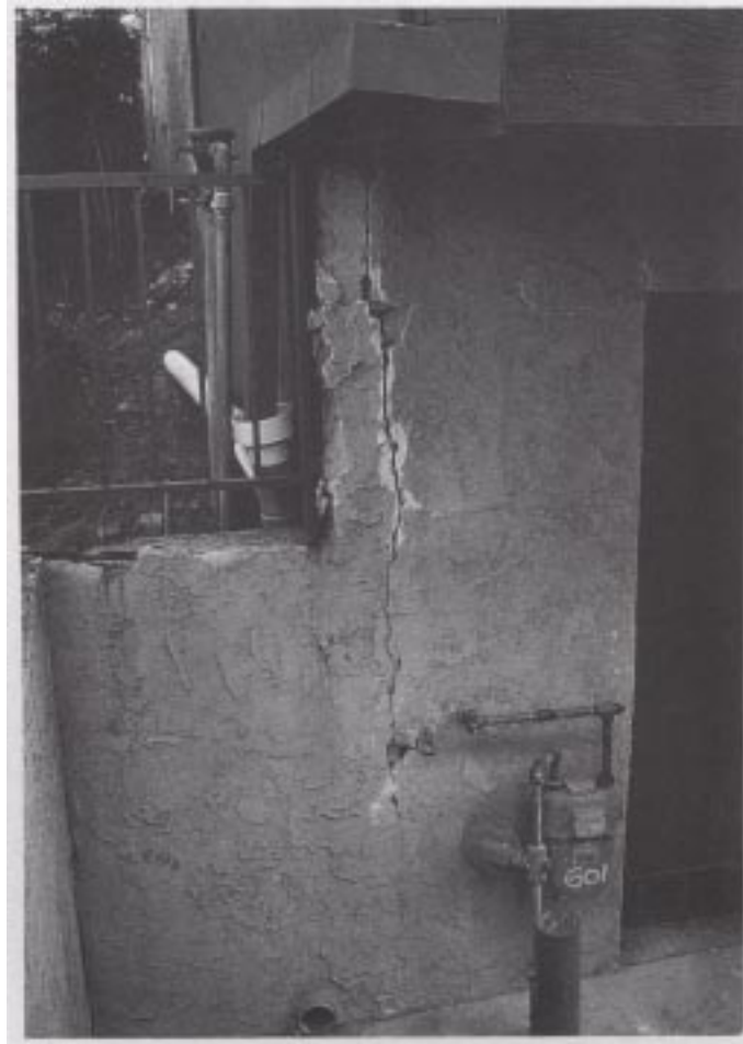
Figure 46. Racking of wood-frame and stucco walls along the garage openings of a SFA building.
