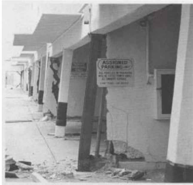
Figure 44. An example of severe deflection of a steel column and stucco shear wall of soft-story MFLR construction.
