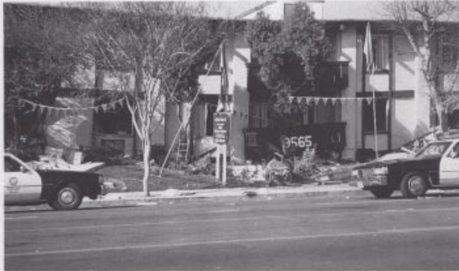
Figure 40. The Northridge Meadows collapse where 16 lives were lost in dwelling units located on the crushed soft story of this MFLR building.
