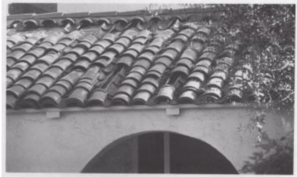
Figure 26. An example of dislodged roof tiles caused by ground shaking and poor attachment.
