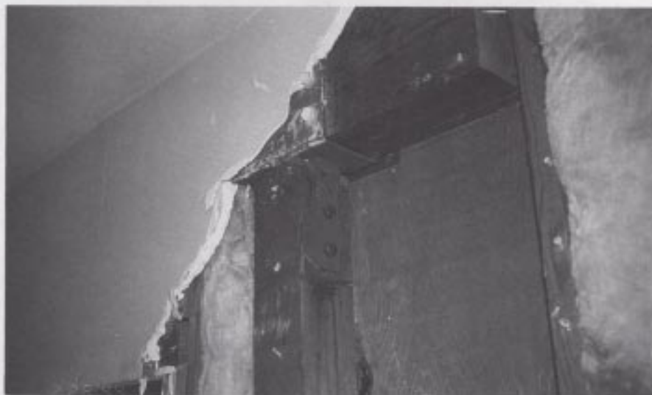
Figure 58. Exposed heavy-timber framing and steel bracket on the first floor showing evidence of a discontinuous connection between the top plate and a header beam.
