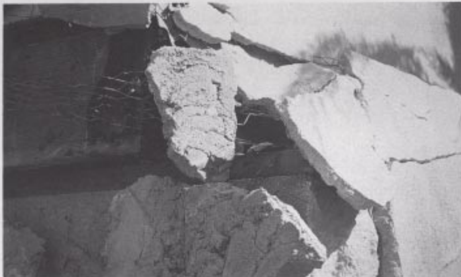
Figure 52. Sliding of floor framing on a crawlspace foundation (concrete stem-wall type) supporting an older MFLR building.
