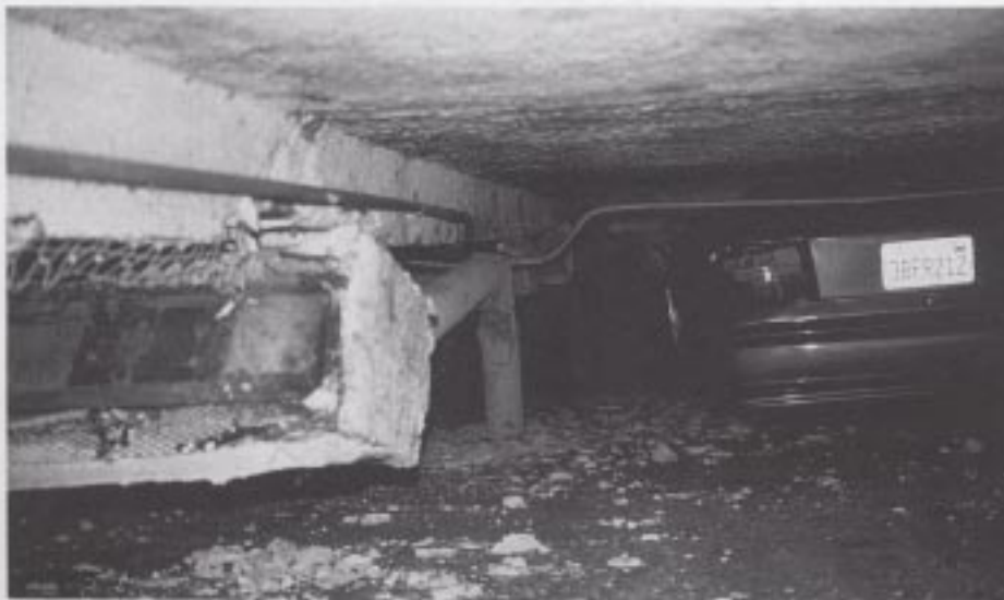
Figure 43. A view beneath the Victory Boulevard MFLR building collapse showing the bent steel pipe column and a crushed vehicle.
