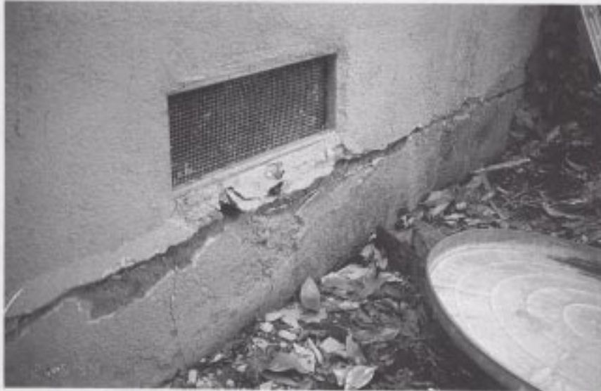
Figure 7. Photograph showing an example of "HIGH" damage to the foundation-wall/floor connection on the crawlspace foundation in a SFD home.
