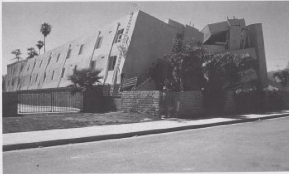
Figure 47. A new (1988 vintage) MFLR building on Sherman Way with a rare collapse of a reinforced concrete and masonry garage foundation.
