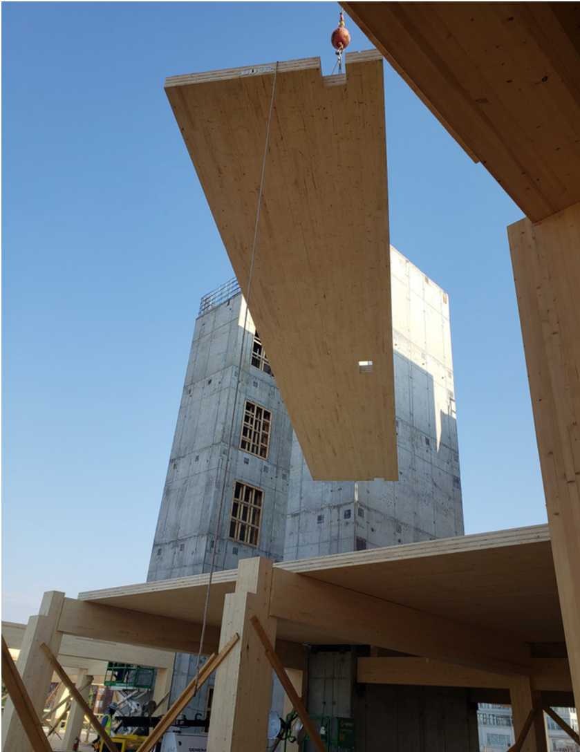
A mass timber panel is lifted into place during construction. Apex Plaza, n.d. Photo credit: American Wood Council (2022).
