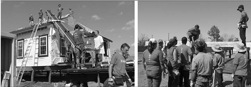
Construction work in progress at 2310 and 2314 Delery Street in the Lower 9 neighborhood, New Orleans, Louisiana. Photo credit: Marsha Cuddeback.
