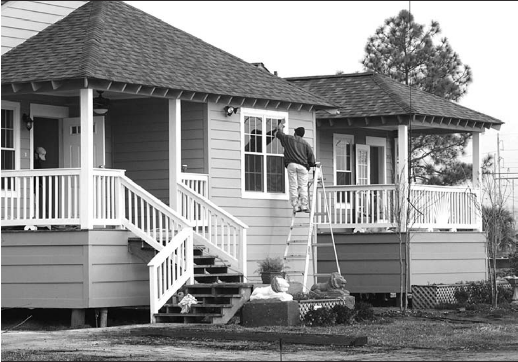
A worker adds finishing touches to completed houses at 2310 and 2314 Delery Street in the Lower 9 neighborhood, New Orleans, Louisiana. Photo credit: Marsha Cuddeback.
