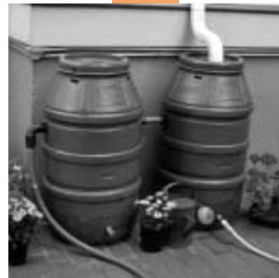
Fig. 4-43a and Fig. 4-43b Rain barrels used to capture rainwater from roofs. Rain barrels can be connected to provide more storage capacity.
