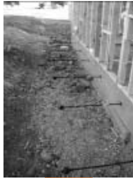
Fig. 4-10 Post-tension slabs-on-grade were used for homes in a rural subdivision with poor soil in Arizona. Life Rebuilders, Superior, AZ
