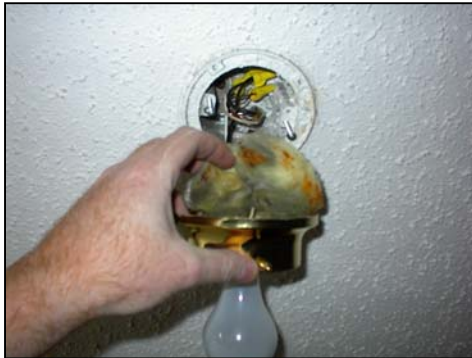
Figure 3-6. Rust on light fixture.
