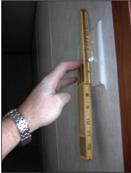
Figure 3-2. Bowing wall near the front door light switch
