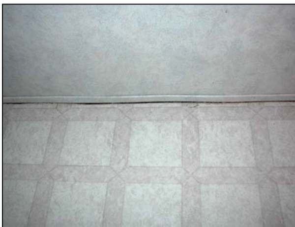
Figure 3-4. Bowed wall seen along floor.
