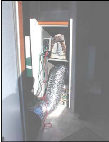
Figure 4-7. Duct leakage apparatus connected to air handler
