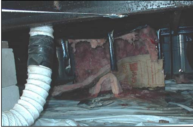
Figure 4-12. View of crawlspace showing damaged bottom board
