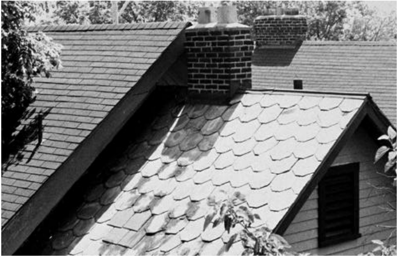
This slate roof should be carefully investigated since it has a makeshift repair. Other problems include the chimney, which is too low, and the vent pipe, which is too narrow.
