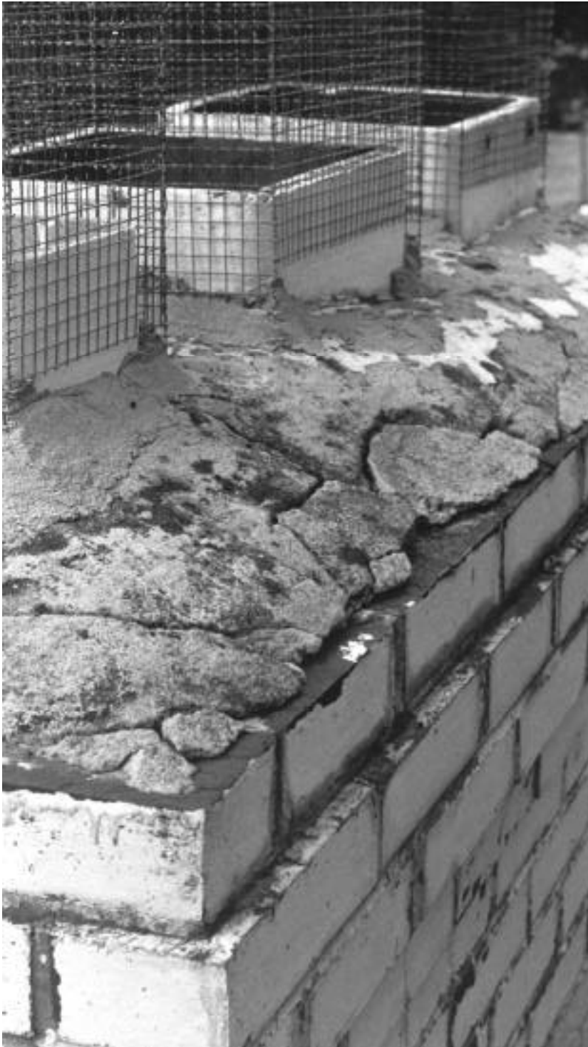
A deteriorated chimney cap. Mortar, rather than concrete, is often improperly used (as it was here) to cap the chimney. The masonry below will eventually deteriorate unless the cap is replaced.
