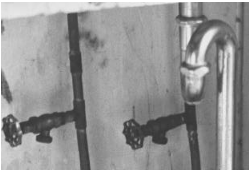
An S-trap that can cause self-siphonage and loss of the water seal. All such traps should be replaced.
