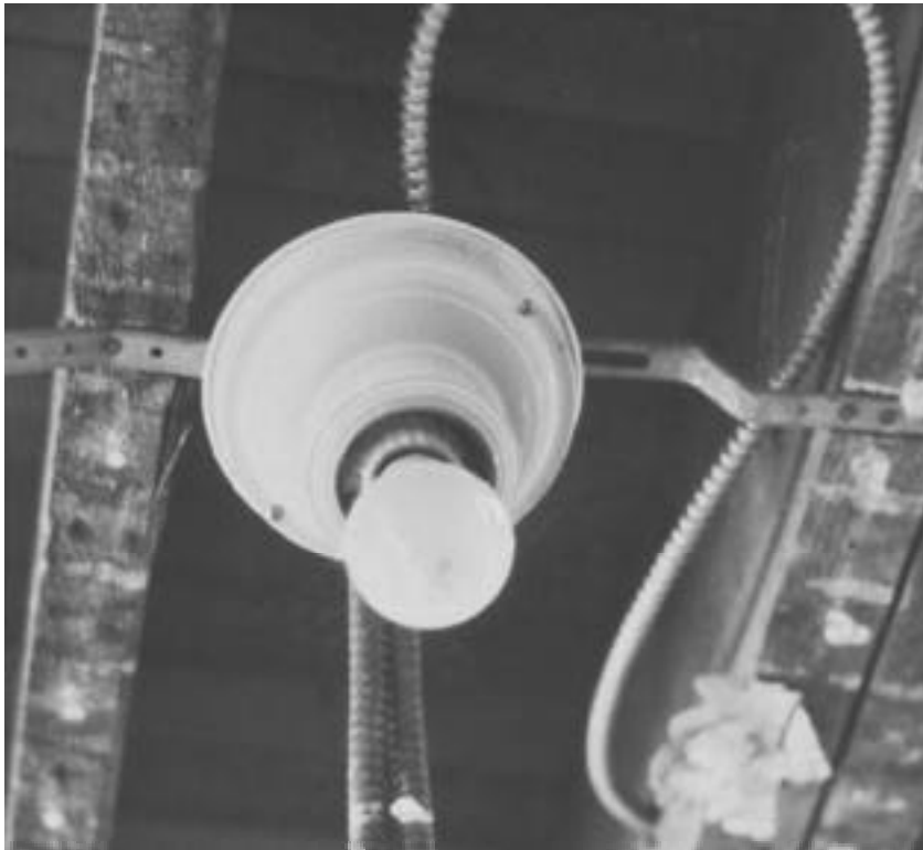
The armored cable and junction box are in good condition and can be reused, even if the lighting fixture is relocated.
