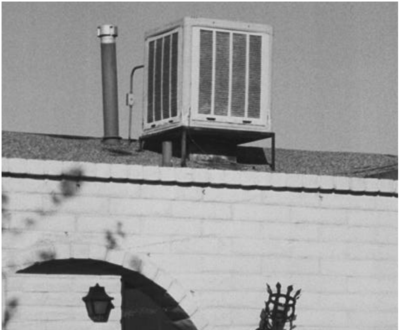
A roof-mounted evaporative cooler. This type of cooling unit is relatively simple to inspect, repair, and maintain.
