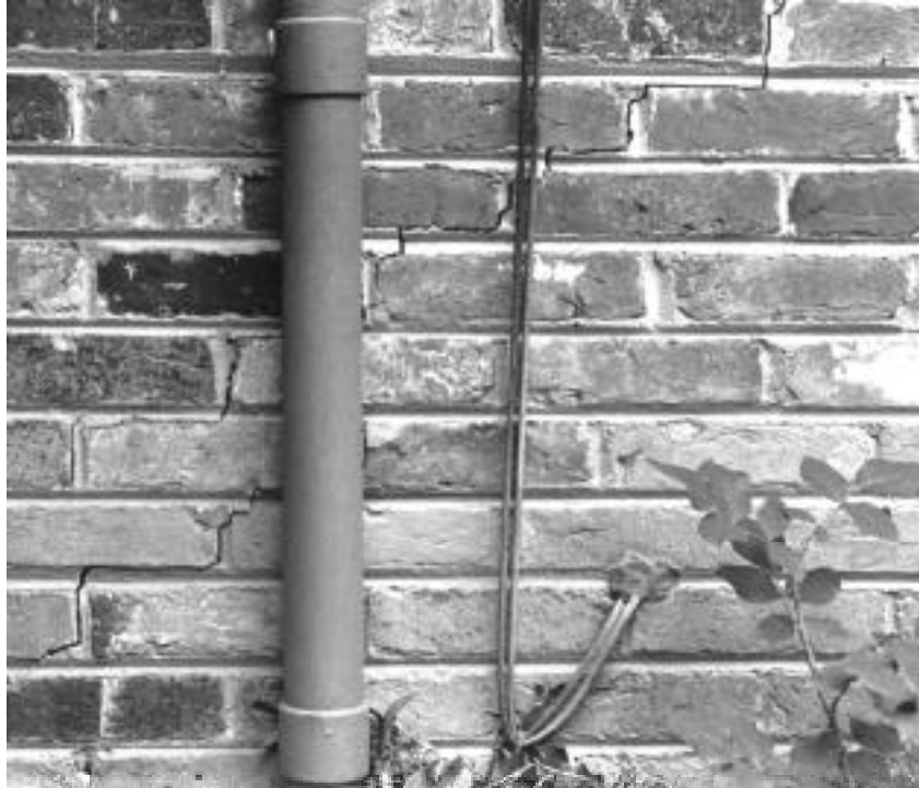
A common masonry wall crack probably caused by thermal or moisture expansion. If possible, monitor such cracks over a period of time to see if they're active. Active cracks should be sealed with a flexible sealant; inactive cracks may be pointed.
