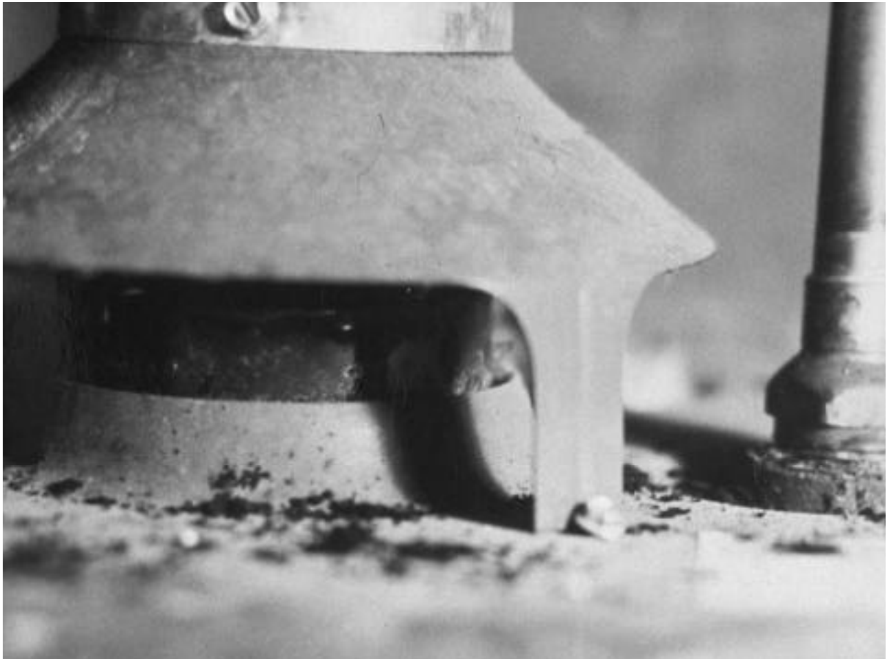
The soot that has accumulated below the draft hood of this water heater indicates a severely clogged flue or chimney, or more commonly, back-drafting caused by insufficient make-up air.
