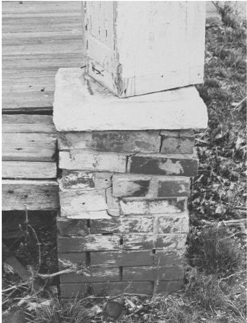
This pier has been overstressed by movement of the porch and column. The entire assembly should be rebuilt.
