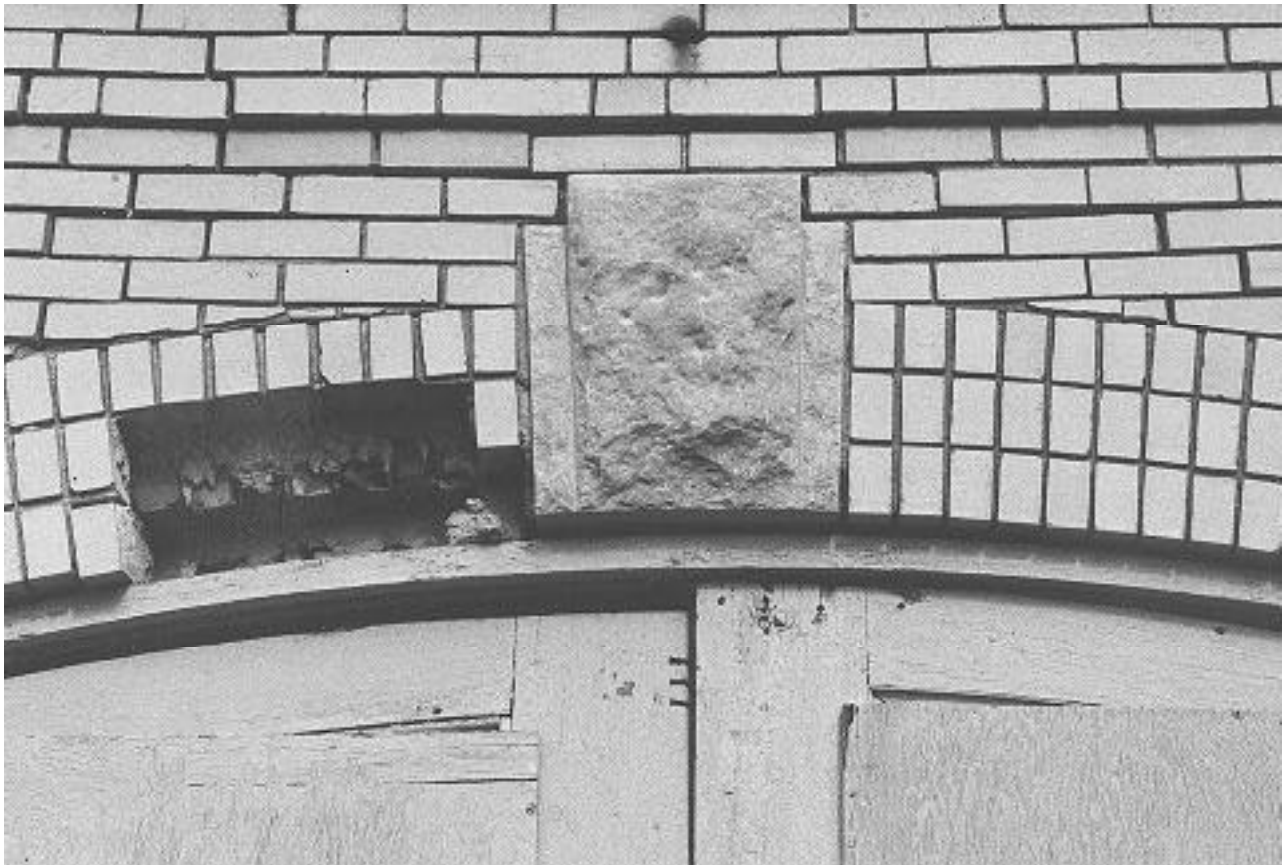
Despite the loss of masonry, this arch is intact and can be repaired with matching bricks.
