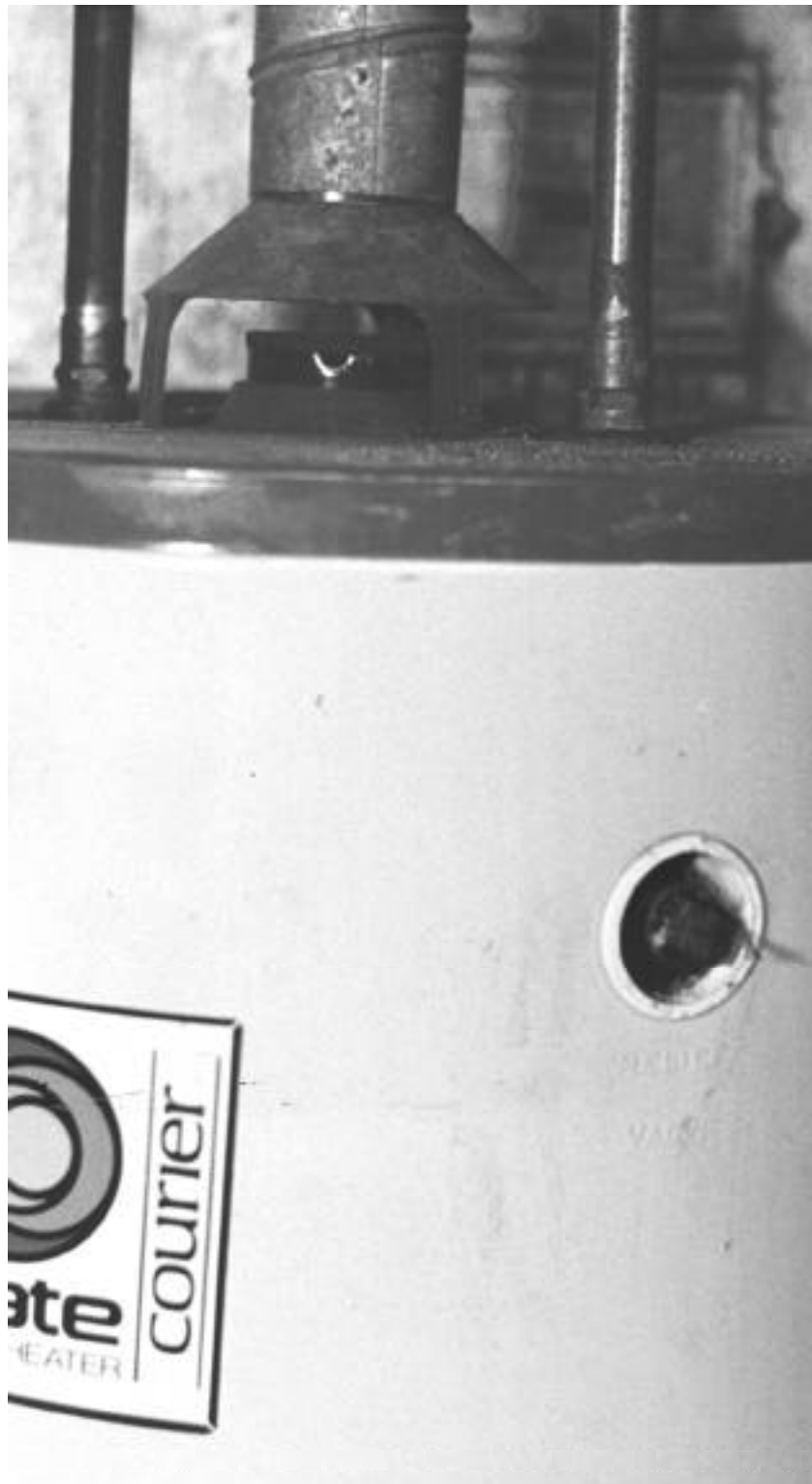
This water heater tank had a threaded plug where its temperature-pressure relief valve should have been, an unsafe condition that should be corrected immediately.
