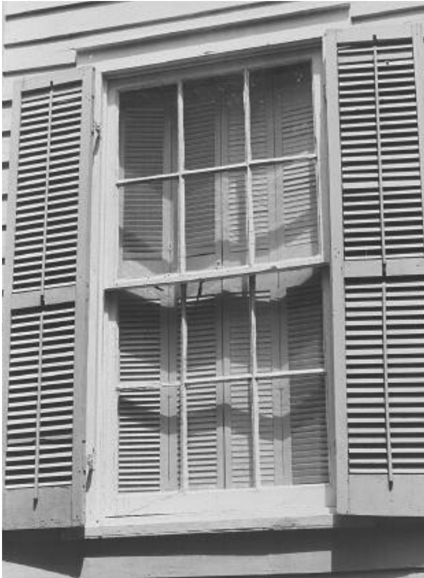
The glazing putty in this window is deteriorated in some locations. Repairs will be time consuming.
