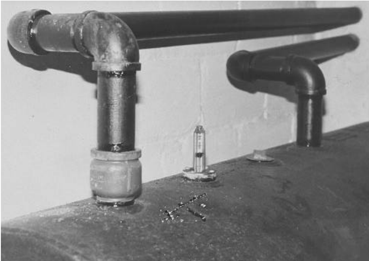
Look for signs of corrosion around and within oil storage tanks and check the operation of the oil level gauge. Use a dipstick to check for signs of condensation in the tank.
